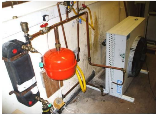
Fig. 15. Shows the connections of the heat exchanger, water pump, heat rejection fan and expansion valve.
