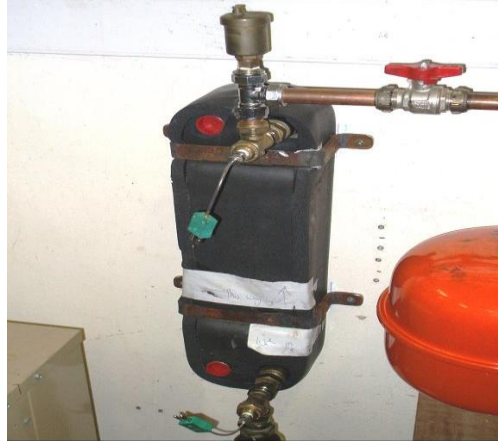
Fig. 14. Shows the heat exchanger.
