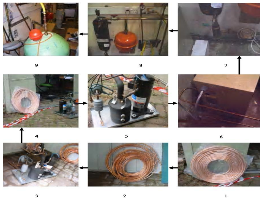
Fig. 4. Showing preparation of coils (1-2), installation of heat pump (3-6) and connection of water supply system (water pump, flow metre, expansion valve and the boiler) (7-9).
