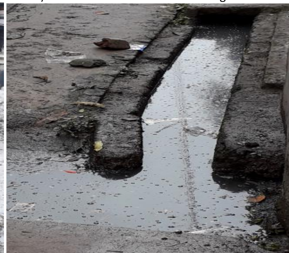
f) Water logged drain
