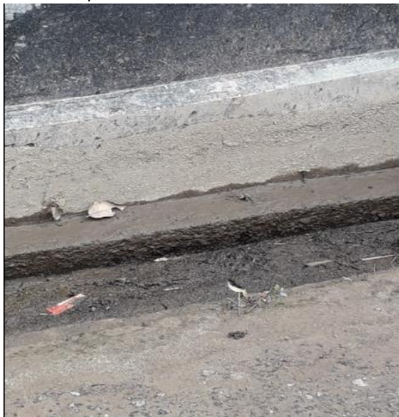
k) Accumulation of sludge blocked the drain completely
