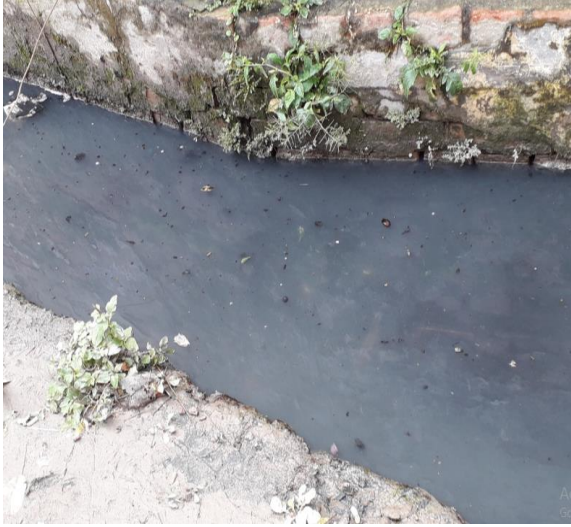
g) Irregular width of drain
