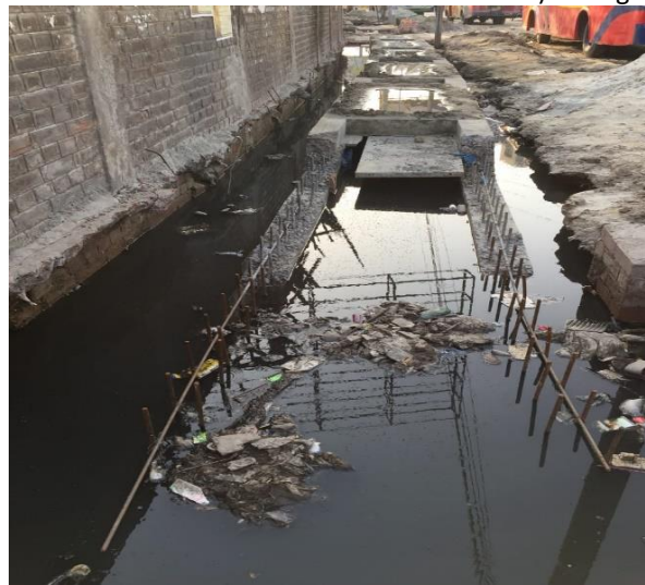
e) Drains under constructions are also vulnerable to waterlogging Fig. 5. Field visit to 3 rd phase drainage development of Rajshahi city.
