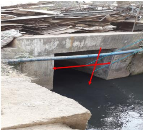
b) Secondary drain (Bhodra)
