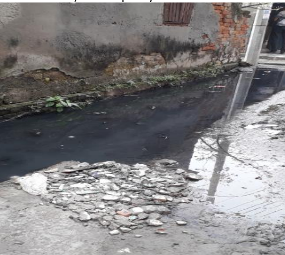
e) Over flowing drain
