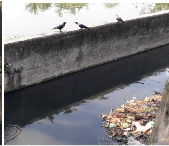
j) Accumulation of solid waste inside open drain
