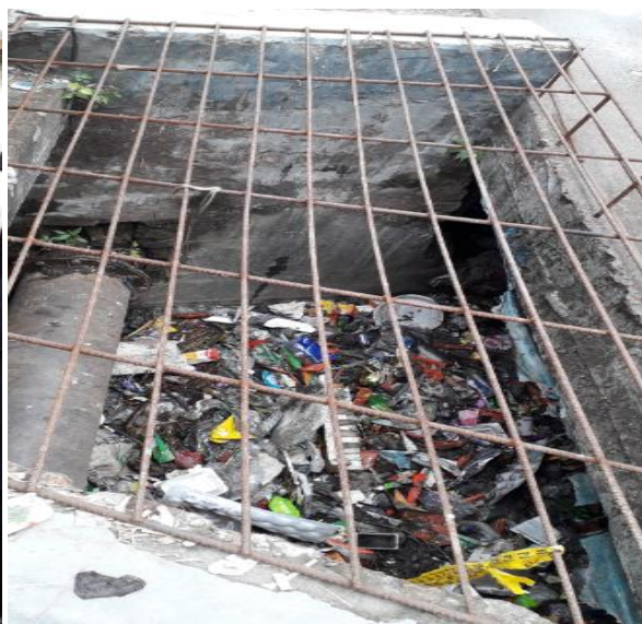
d) Accumulation of waste at drainage bend
