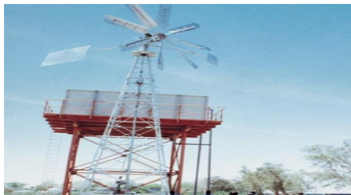
Fig. 8. Locally-manufactured wind pump installed at kilo 8 site.
