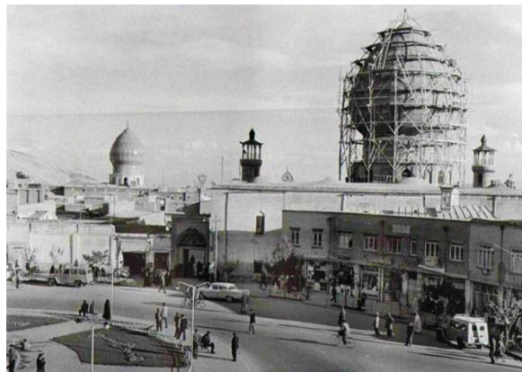
Fig. 4. This picture was taken from Ahmadi square and repairs dome is visible in the photo well.
