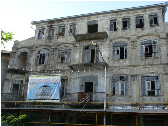
Fig. 8. the repair of historical building of Ministry of Justice in Anzali Port.
